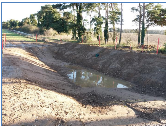
Figure 4. Silt trap (1) installed in December 2017.
